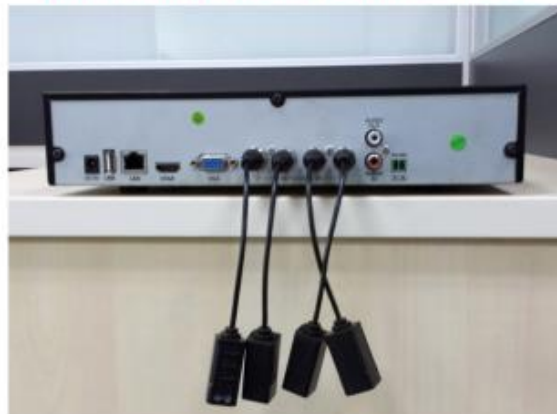
Old baluns make the cabinet a mess
